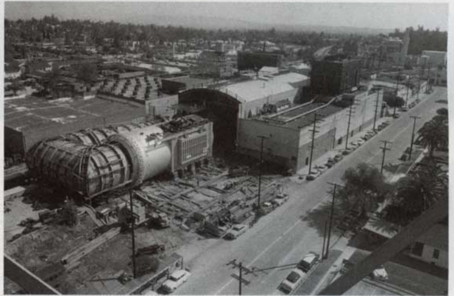
As documented in this historic photograph, the turbine was removed from the wind-tunnel building for a rare cleaning.
